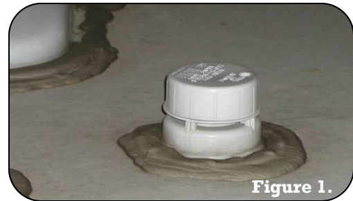
Unsightly "caulk" prone to cracking & leaking
